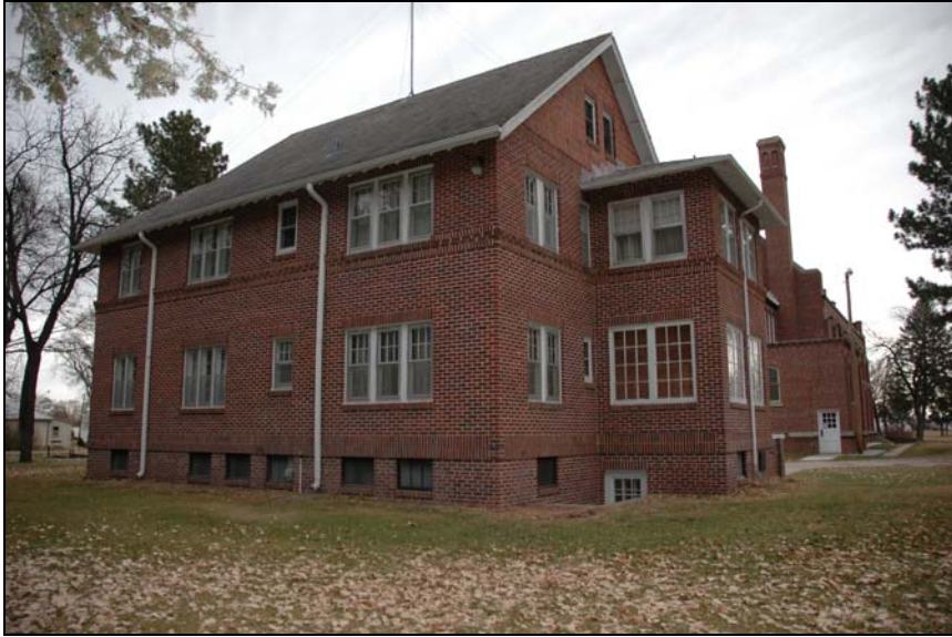
St. Anselm's Church, Rectory & Parish Hall Photo by Stacy Stupka-Burda Photo 8 of 12 – View of rectory, W façade, looking E
