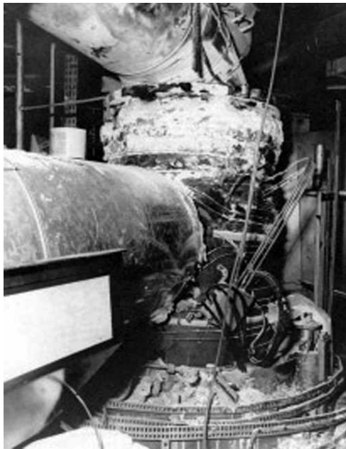
Figure 2.7 Phénix heat exchanger with insulation removed after sodium fire. Photo: Sauvage, 2004
