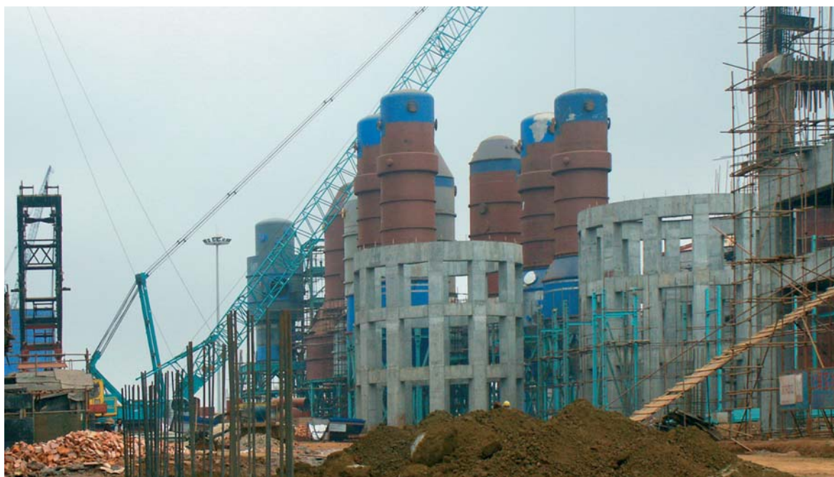
The greenfield Hainan Jinhai Pulp & Paper Co., Ltd mill, sited in the Yangpu Economic Development Zone on the island of Hainan in the South China Sea, is scheduled for start-up in the autumn of 2004.
