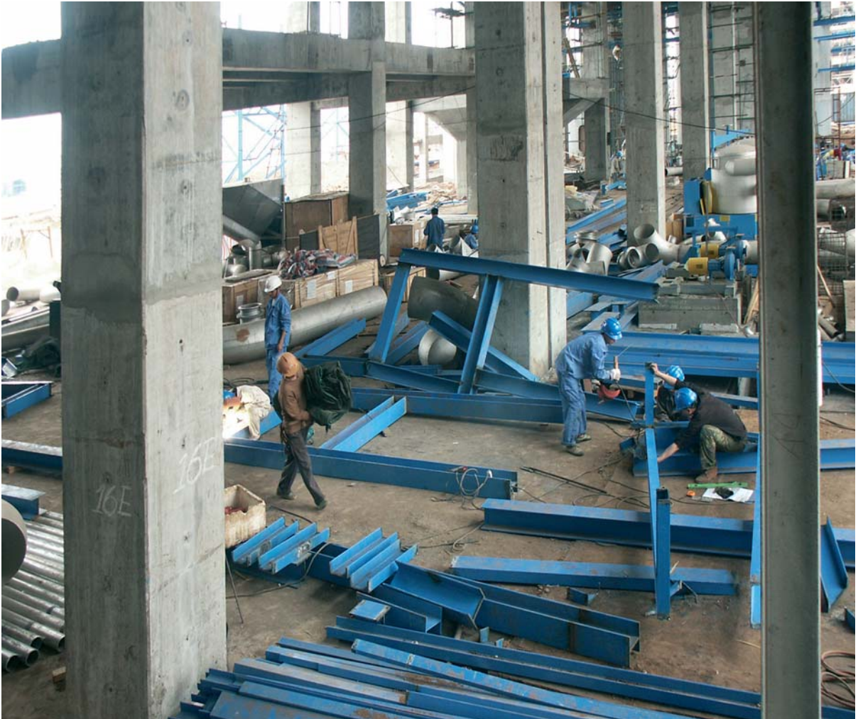
Work at the Greenfield mill site is intensive in anticipation of meeting the scheduled start-up.
