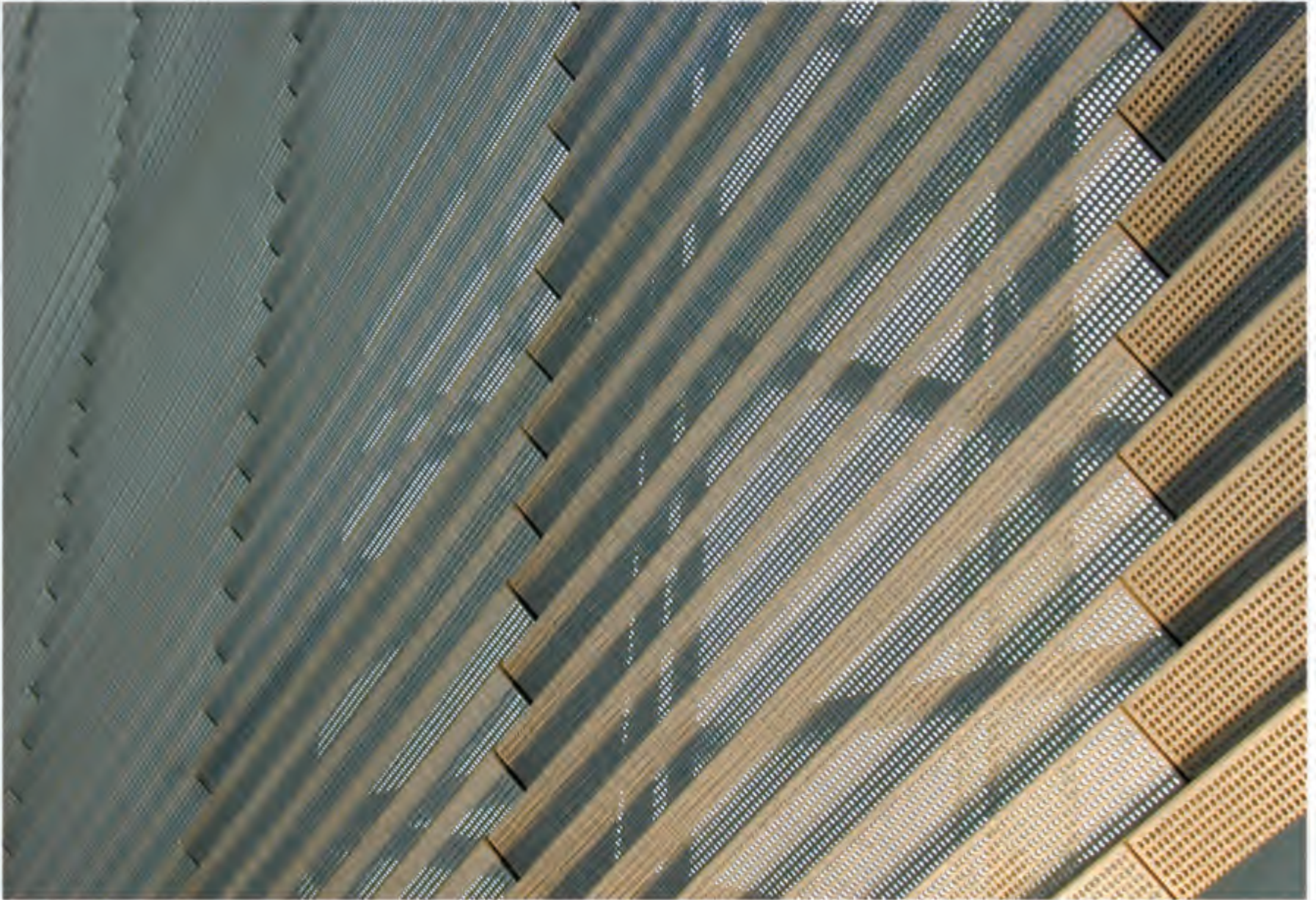
The Nerman Museum of Contemporary Art - Kyu Sung Woo, Architects. Custom, perforated and pleated aluminum louver sun screen system.
