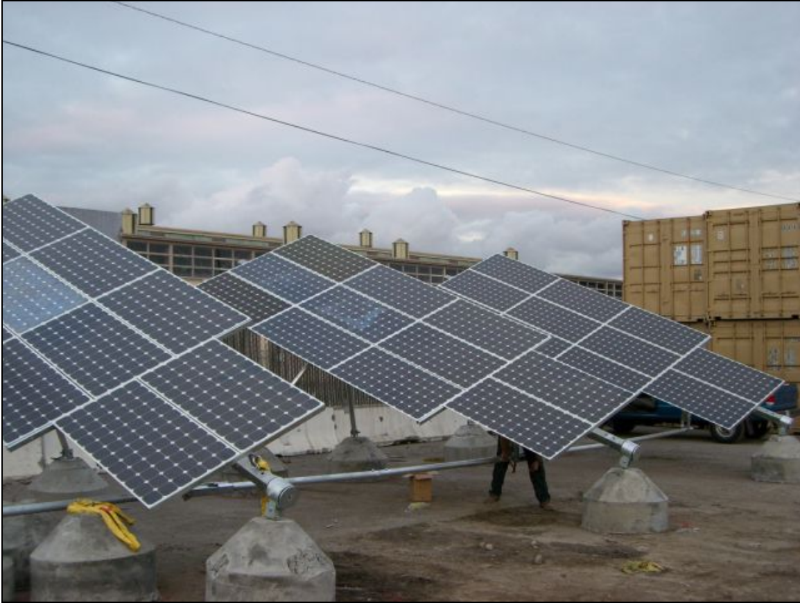
Figure 38: Installed Prototype System
