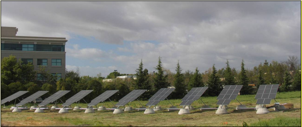
Figure 26: Prototype T20 tracker installation in San Jose, California.
