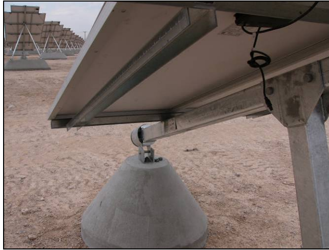
Figure 31: One of two struts to protect PV from collision with drive strut
