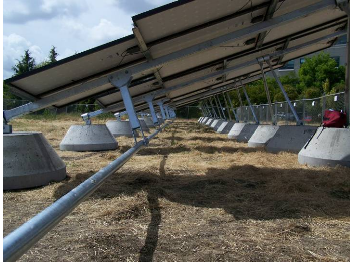
Figure 28: Drive strut connecting multiple T20 units
