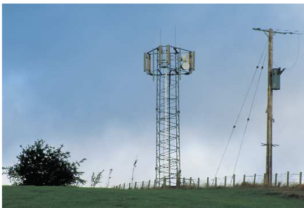
Telecom mast in prominent location, near Haugh of Urr
