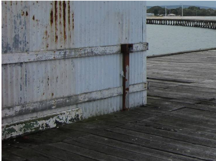
Figure 30: Join between the decking beneath the slipway shed and that on the surrounding deck, suggesting that the latter has been replaced more recently.
