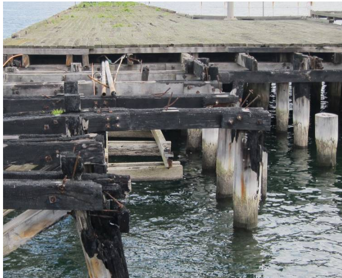
Figure 34: Remains of the original low landing (centre of the picture) beneath the 1982 extended turning bay.
