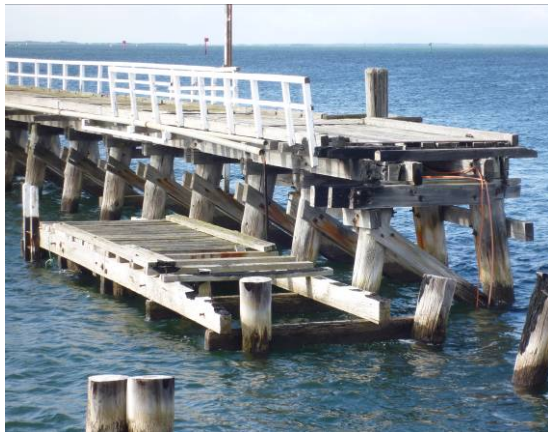
Figure 37: 1982 low landing today, having been damaged by the 2010 fire and partially dismantled.
