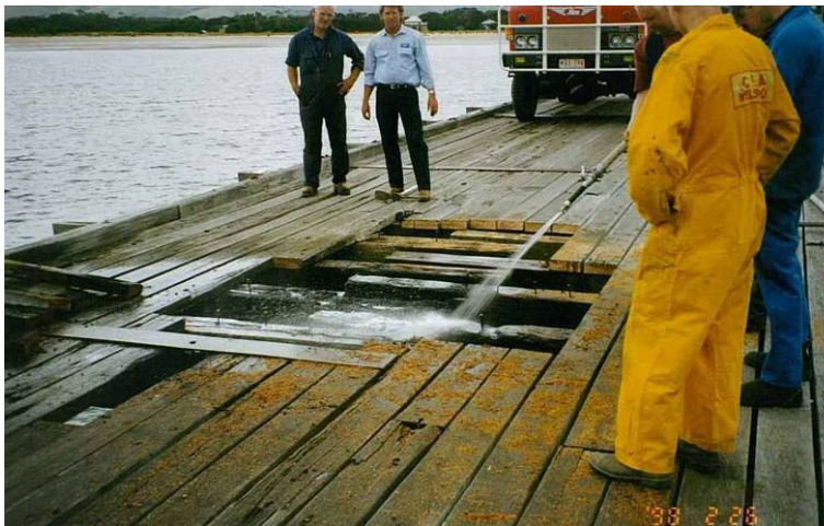
Figure 23: Damage to the jetty decking and transoms after a fire in 1998.
