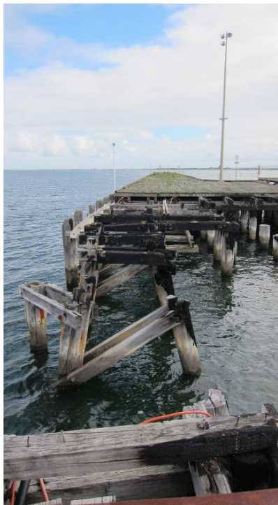
Figure 26: The pile bents of the original approach extending towards the original loading area. The surviving piles of the 1982 extended turning bay can be seen to the right.
