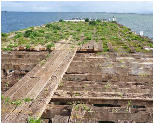
Figure 40: The 60m extension today having deteriorated significantly.
