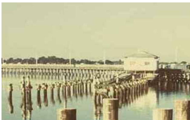
Figure 27: The slipway section in 1982. This would appear to show the slipway during its dismantling as the decking of the finger jetties has already been removed but the crossheads can still be seen at the tops of the piles.
