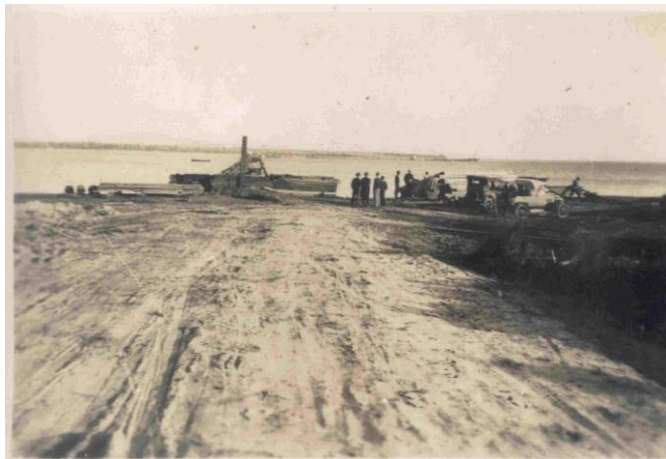
Figure 5: The site of the Long Jetty is prepared (photo source: Norry Rossitter).
