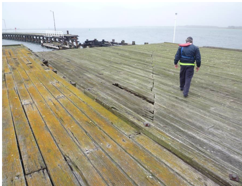
Figure 35: The remains of the extended turning bay showing the planking of the extended area butting against that of the original loading area.
