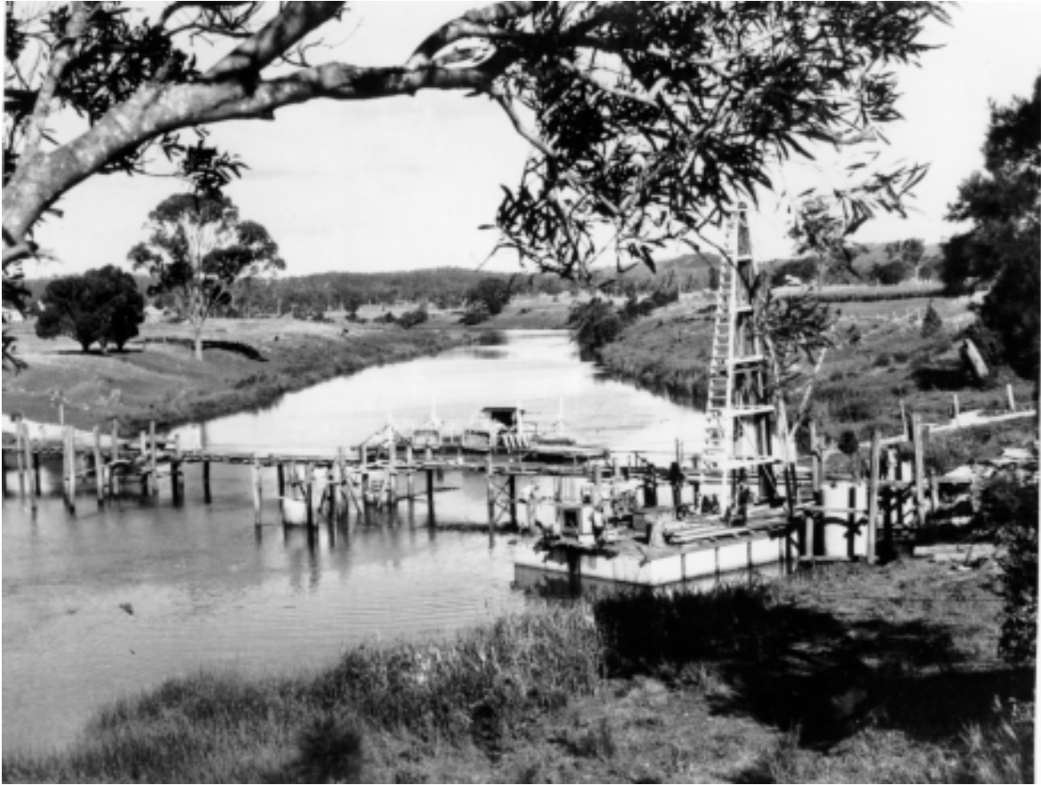
Building a new bridge at Waterford 1954 after the previous one had been damaged in the 1947 flood. The ferry can be seen on the far side. (Source Keith Schmidt)
