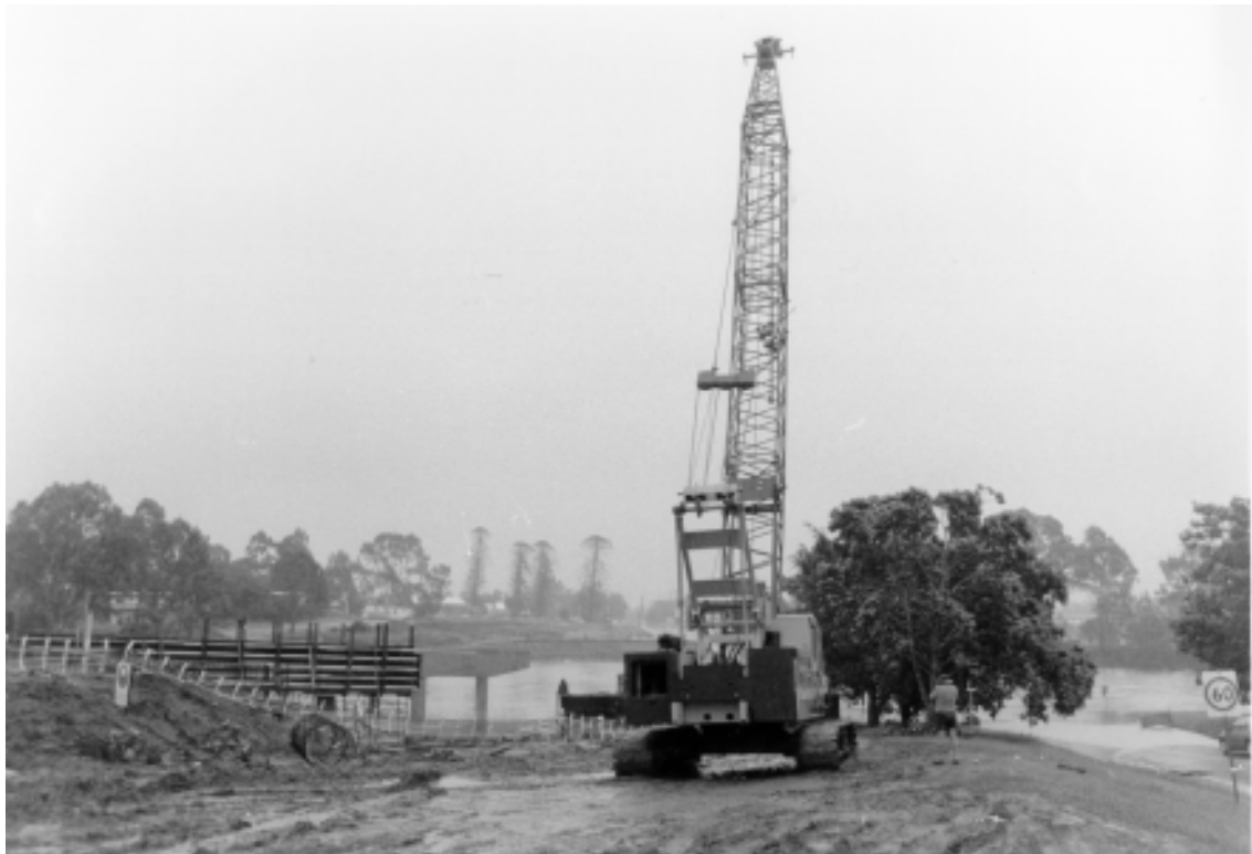
Construction of the high-level Waterford Bridge is delayed by floods in May 1996. Looking towards Waterford West. Note the road leading to the submerged existing bridge. (Source: Keith Schmidt)
