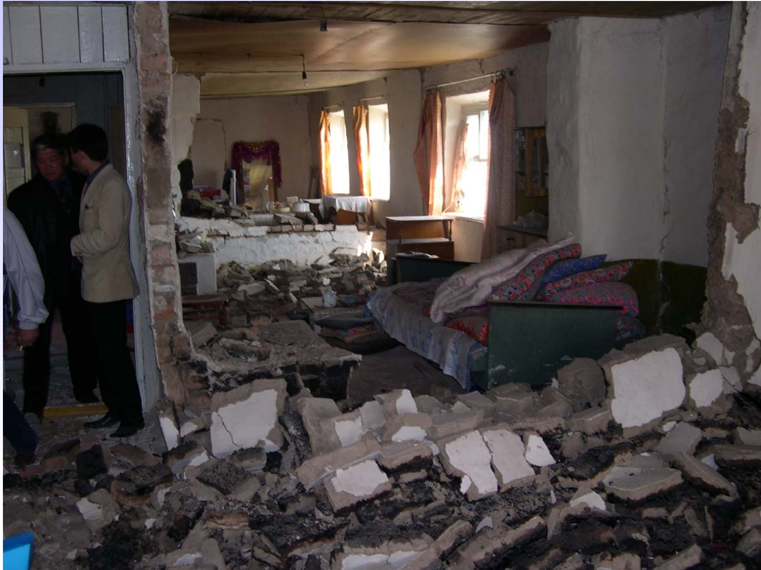
THE 26.04.2008 SHALKARSKOE EARTHQUAKE - Destructions of buildings
