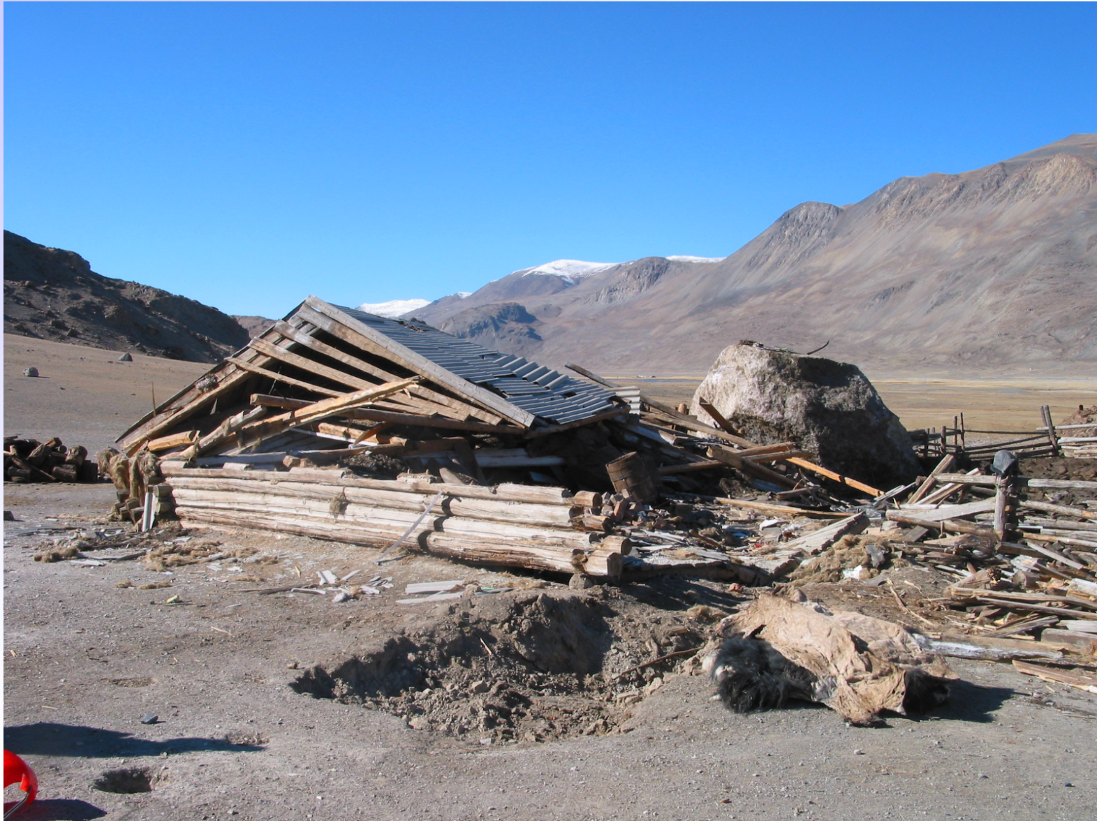
THE 27.09.2003 MOUNTAIN ALTAI EARTHQUAKE - The shepherd house in the valley of the Taldura river, destroyed by falling of a stone
