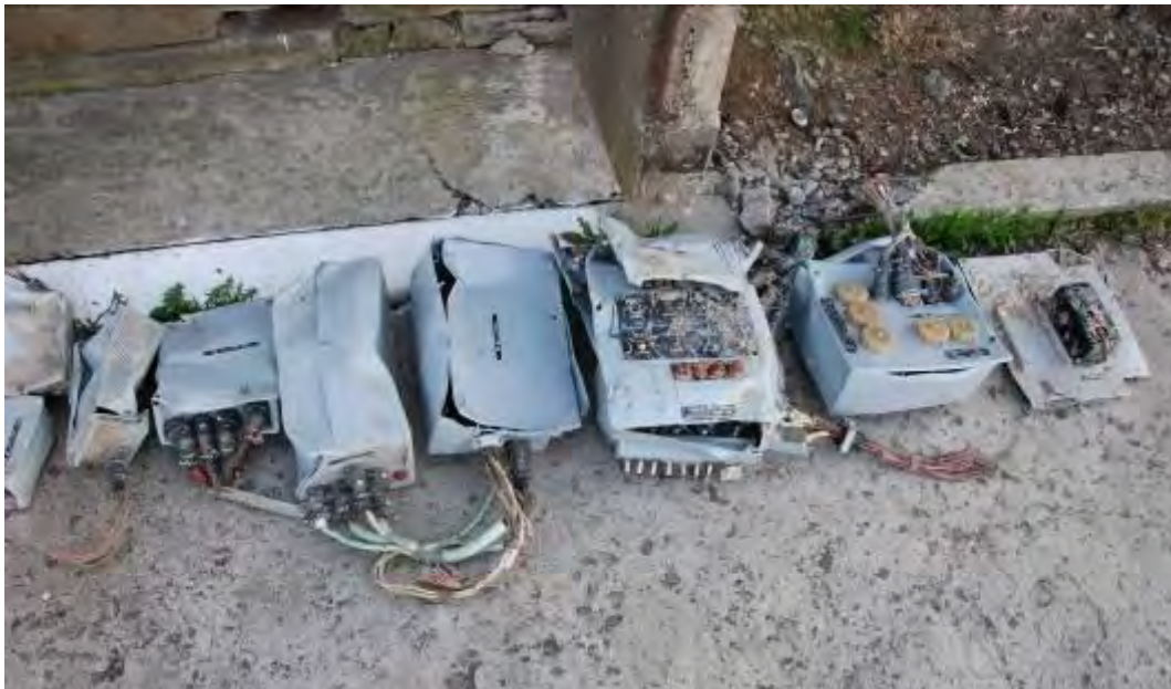
Fig. 30. The control boxes of the electrical system
