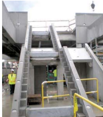
An unfinished staircase and escalator at the Wiehle Avenue Silver Line station.
