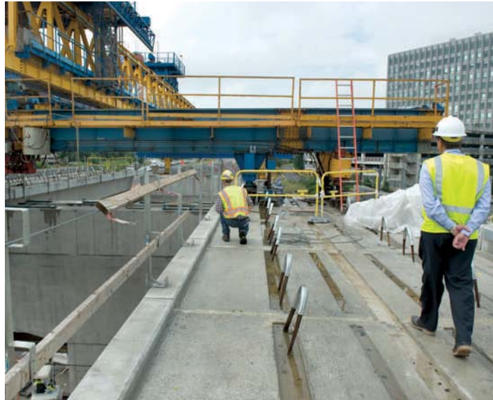
Metro crews work on the Dulles Corridor Metrorail Project in Vienna last September.
