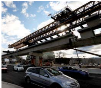
Crews work on the Silver Line in Tysons Corner in McLean, Va., in November 2011.
