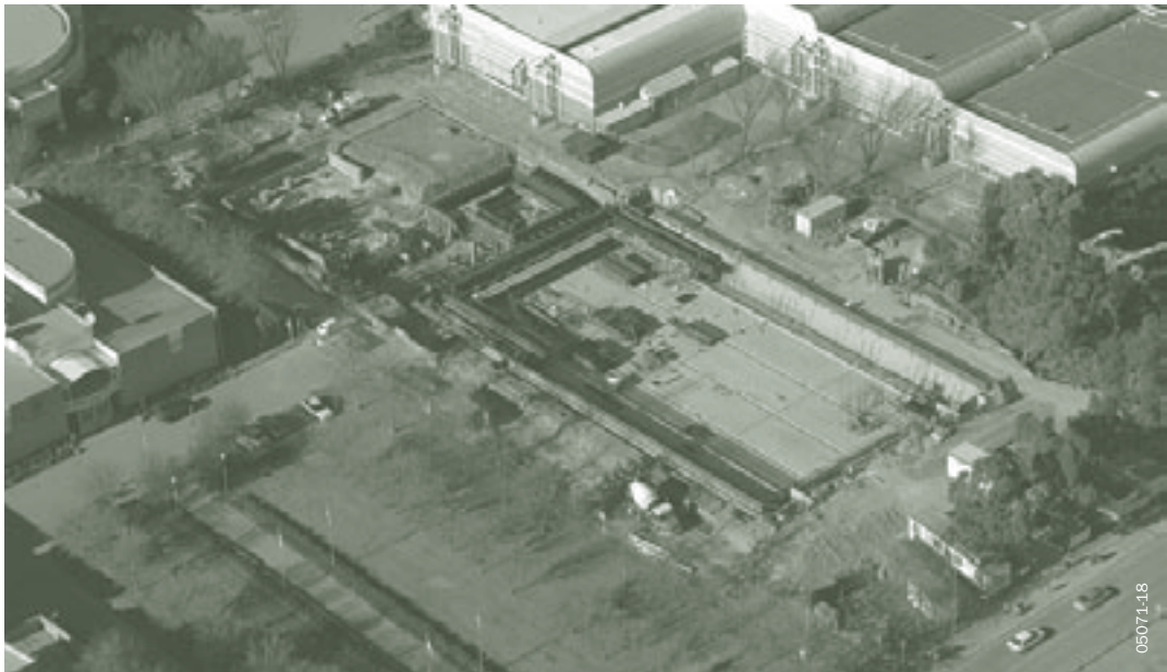
An aerial view of the construction of the aquatic testing and training centre, Australian Institute of Sport, 2005
