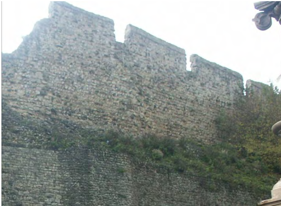
West curtain wall: Norman walling above Roman foundations and 20 th century retaining walls with 18 th century crenelations 11
