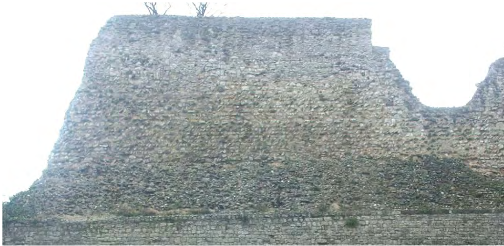
West curtain wall: Norman walling above Roman foundations and 20 th century retaining wall with inserted 13 th century windows
