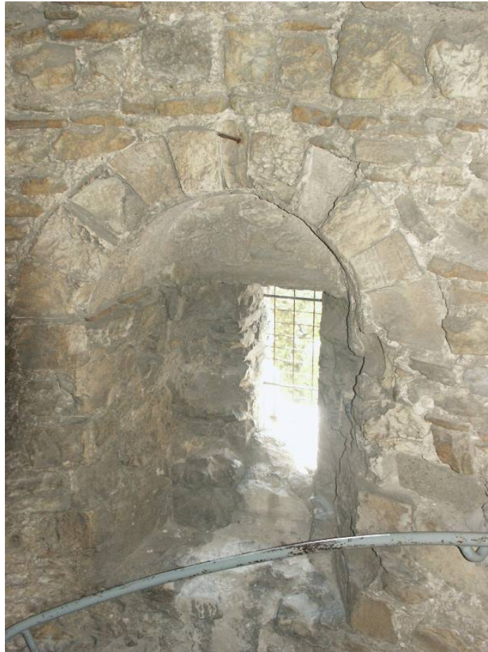
South-west tower: Damage to internal window openings
