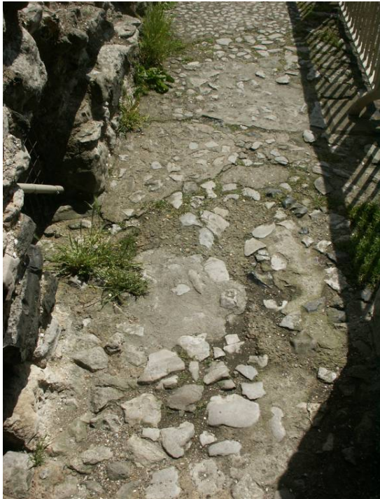
Damaged wall top
