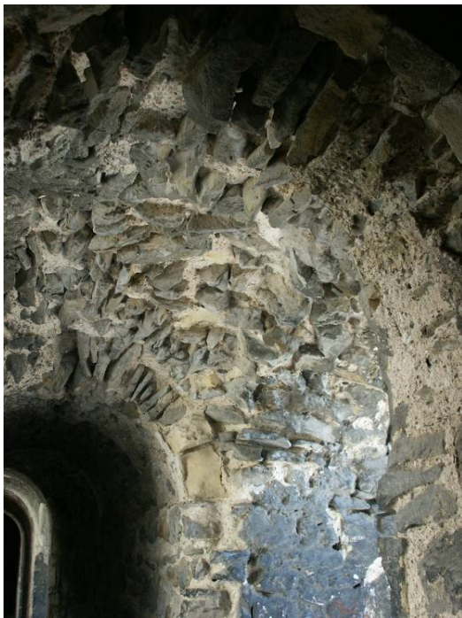
Loss of mortar in the gallery vaults
