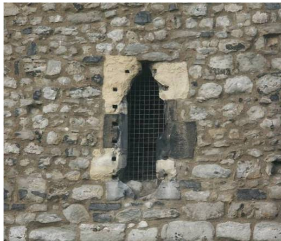
Tower two: eroded window opening
