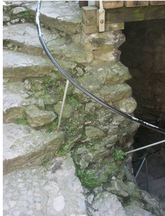
Water ingress through north-east stair
