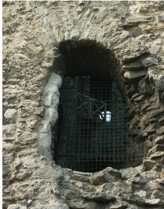
East elevation: incomplete window opening
