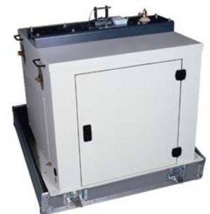
AM Antenna System ATU
