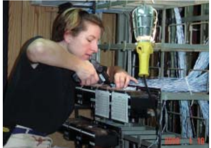
Master Sgt. Valerie Goehring helps connect a 900-pair cable to the SMU.
