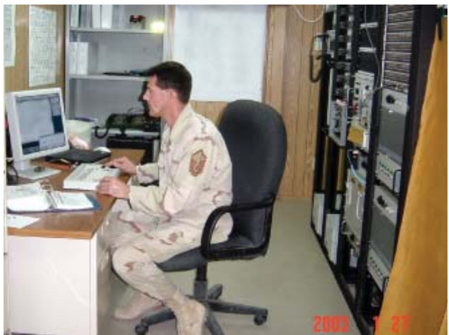
Master Sgt. Andler monitors circuit activity at the operator interface console.
