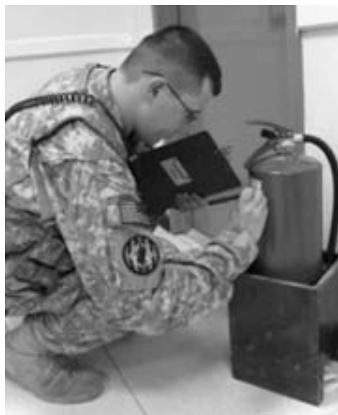
➤ Spec. Zachary Howard completes his monthly inspection of the fire extinguishers, ensuring that safety standards are being met. U.S. Army photos by Spec. Katherine VanAlstine.
