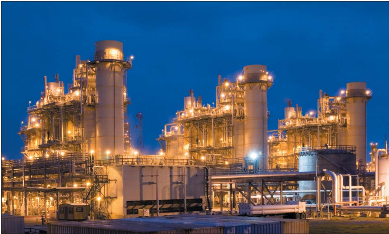
A second and third cogeneration train, each with 160 megawatts of capacity, started up at Beaumont in 2005. Cogeneration is the simultaneous production of electricity and steam. It is up to twice as efficient as traditional methods, and saves energy costs and lowers greenhouse gas emissions.
