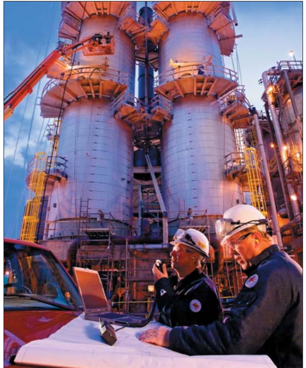
Technicians work to install a new distillate hydrotreater unit at the Joliet, Illinois, refinery, one of several ExxonMobil facilities that will start up in 2006 to produce lower-sulfur diesel for U.S. consumers.
