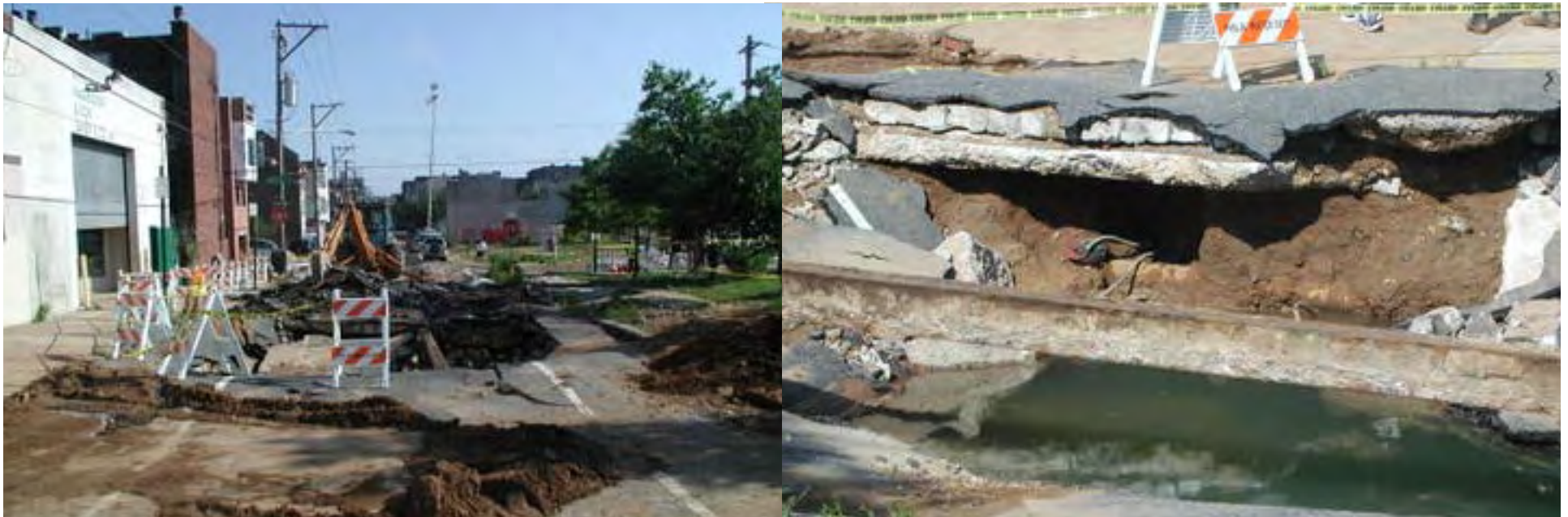
Aftermath of July 22nd, 2005 water main break, 900 block of N. 3rd Street
