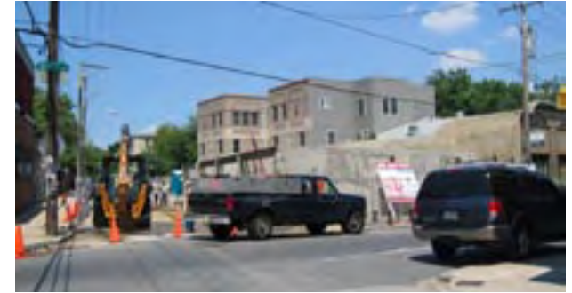
Sidewalk obstruction caused by construction
