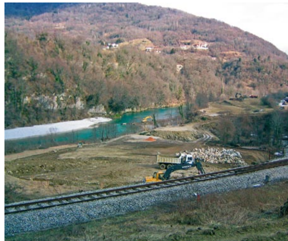
Location of the powerhouse shaft on the terrace of the Soča River
