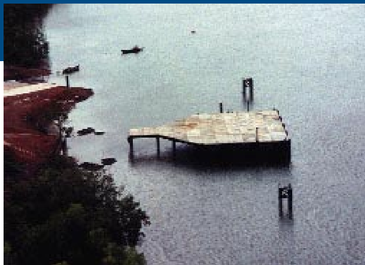
About 1500 T of steel and concrete installed by GEOCEAN in the remote Heinze river near TAVOY, Myanmar.
