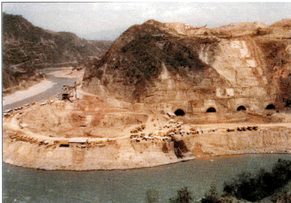
Photo 3: Panoramic view from right bank of Ravi looking upstream ( at the beginning of construction of project), showing Outlet Portals of the Diversion Tunnel and excavation of the Power House pit. The dam axis lies just upstream of Power House location in the left background across Ravi
