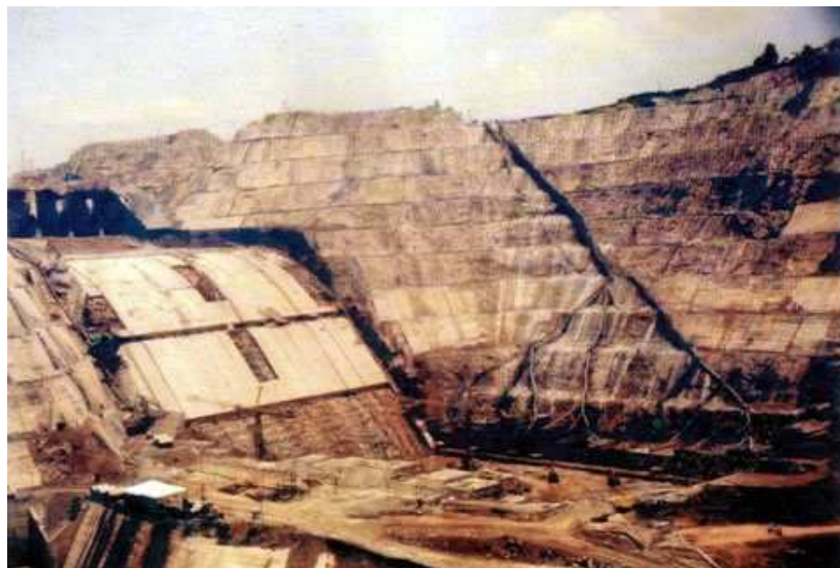
Photo 5: Left flank Spillway construction under progress. Hill-cut benches towards left side, shotcreted and covered with concrete claddings are also seen.
