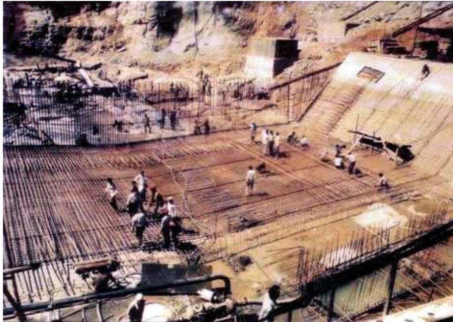
Photo 6: Power House construction under progress. Foundation being designed as raft foundation over rocks of varying competency
