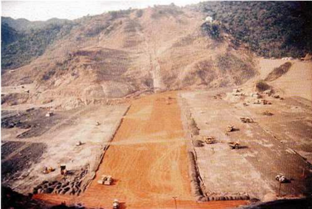
Photo 4: View of Dam looking towards right abutment at higher elevation. Impervious Clay Core flanked by upstream (towards right) and downstream (towards left). Filters and pervious Shell Zones compacted by rollers
