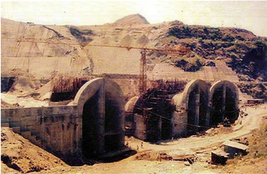
Photo 2: Construction of False Structural Portals at Inlets of Diversion Tunnels in Progress
