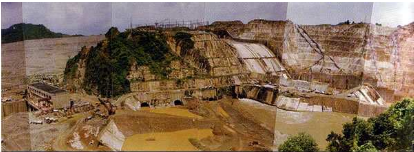
Photo 1: A Panoramic and composite view of Ranjit Sagar Dam Project in final stages of construction (view from right bank of Ravi River)
