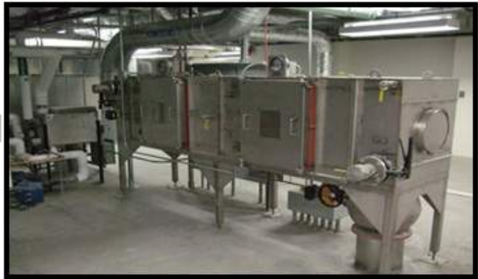
Figure 1-6. HEPA filtration plenum.
