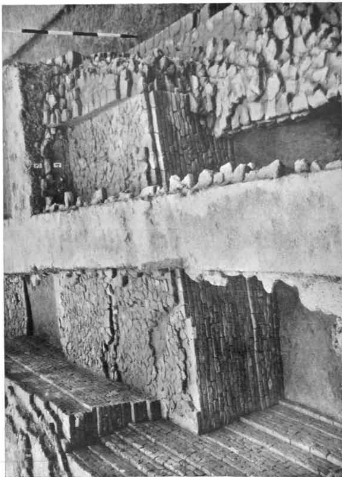
Chandraketugarh : massive brick buttress between main temple and outer structure, Period IV. See p. 64
