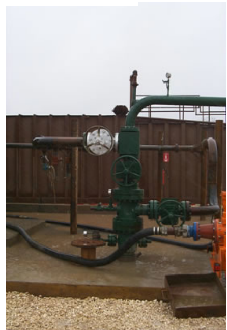
Figure 29: Injection well for cavern
