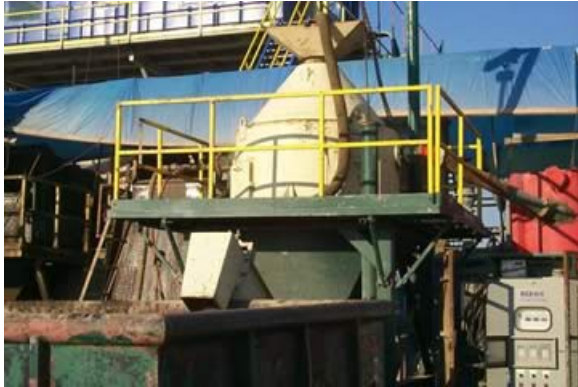
Figure 5: Vertical cuttings dryer
