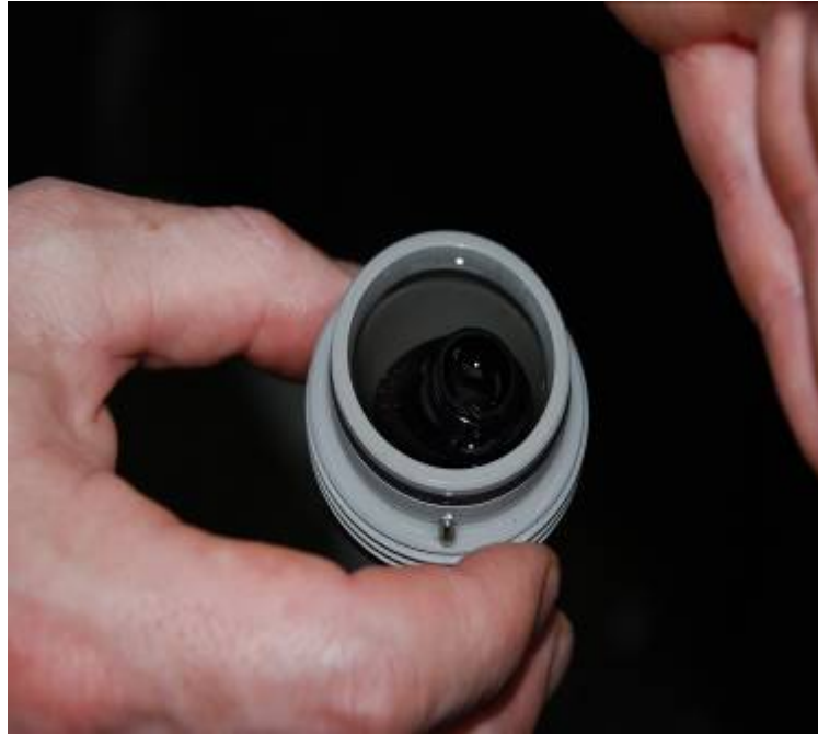
Figure 5: Fuel filter found clean condition
