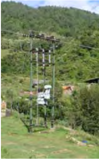
Photo 21: Pole mounted transformer
