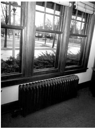
Figure 58 Cast iron hot water radiators in the dining room, under north facing windows. HOBO temperature sensors were taped to the radiator supply and return piping in the basement.
