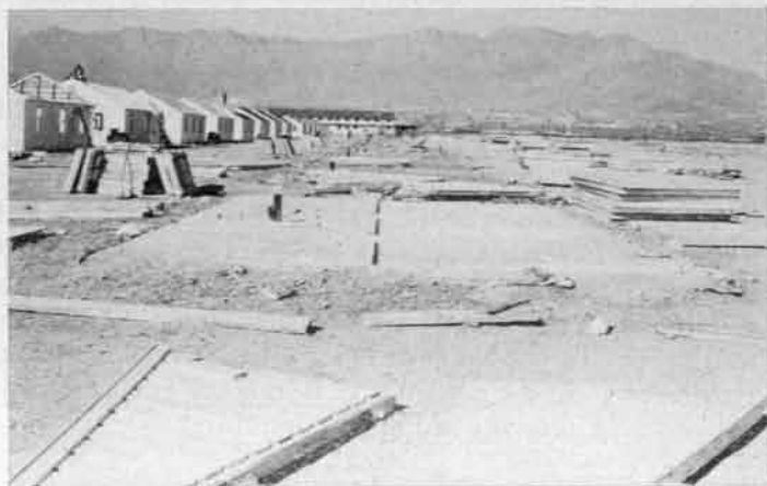
Status of Construction on 2 March 1949. Volunteer Troop Labor Rush Building in Record Time.
