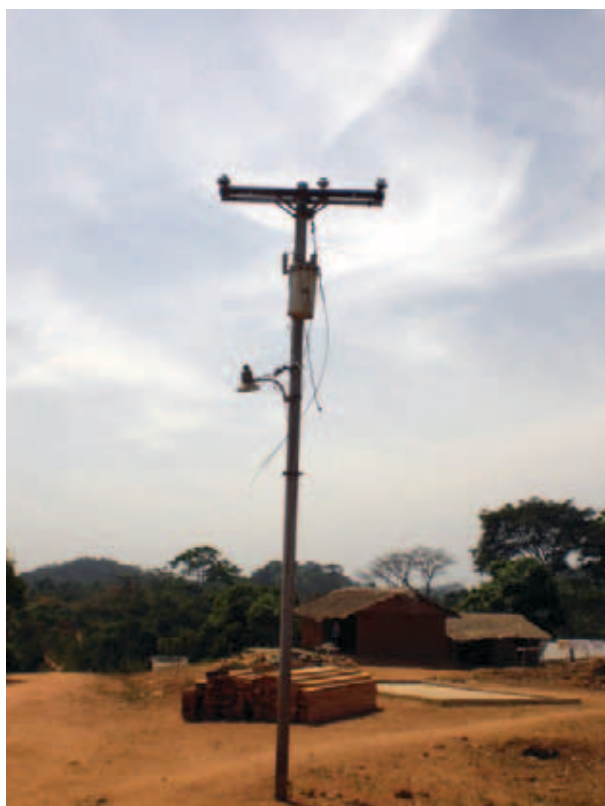
Prewar power pole in Yandohun, Lofa County.
