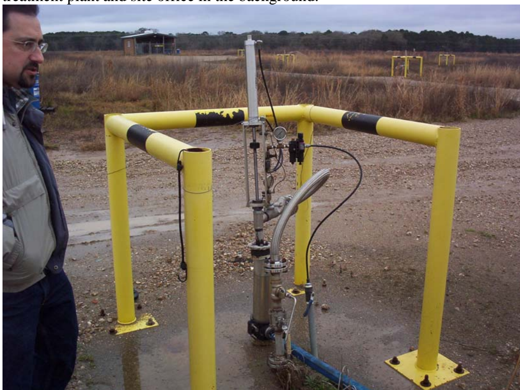
Photo 6. Facing southeast, DNAPL well B07DW in foreground; Hub Facility "C" in the background.
