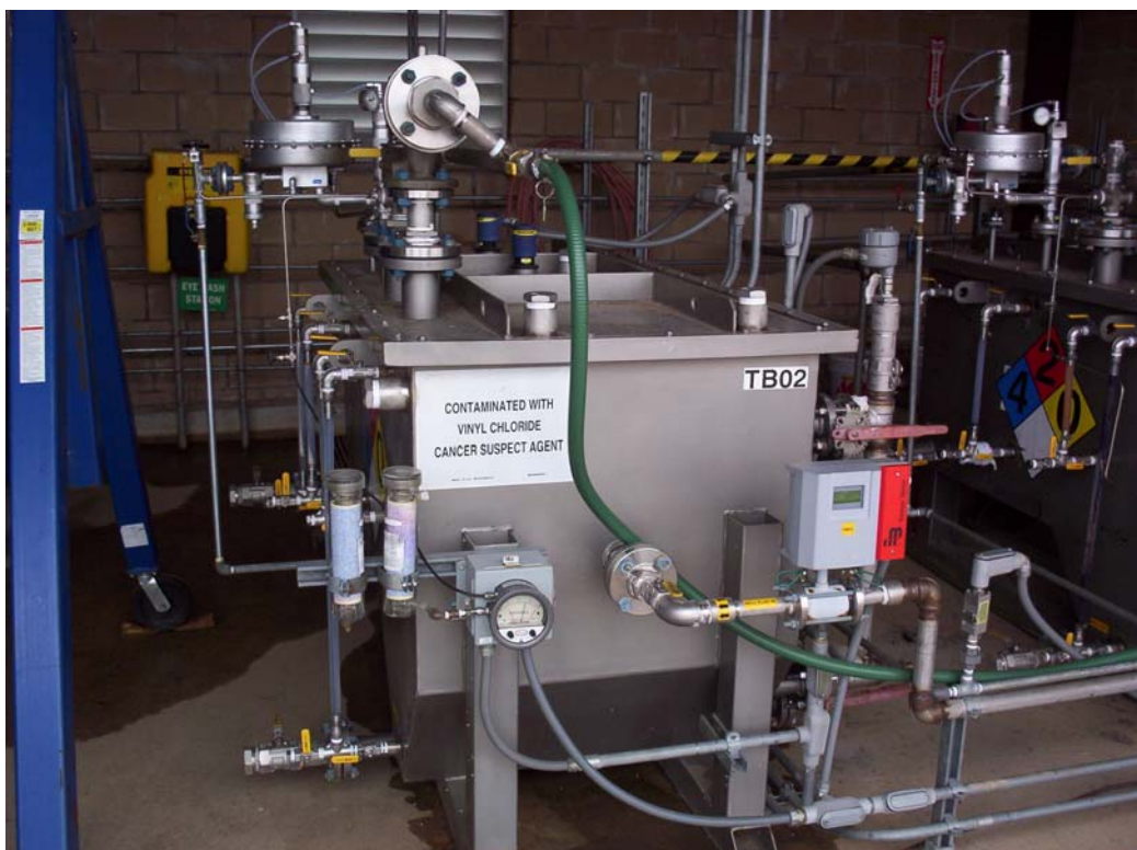
Photo 8. DNAPL/LNAPL separator for groundwater extraction wells in Hub Facility "B". Separator for DNAPL wells located to the right.
