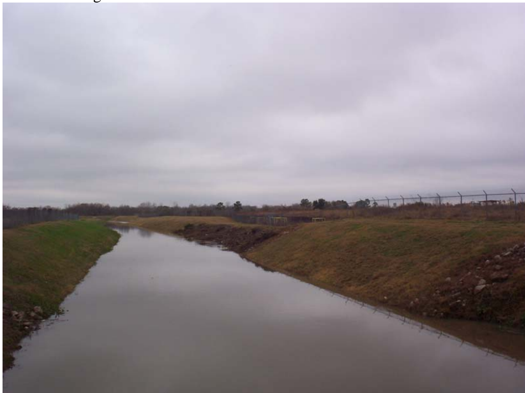
Photo 12. Looking west, upstream on Mud Gully from the Dixie Road Bridge. Note cofferdam wells from Photo 10 in middle right of picture and bank slope creep on side of Brio-North site.
