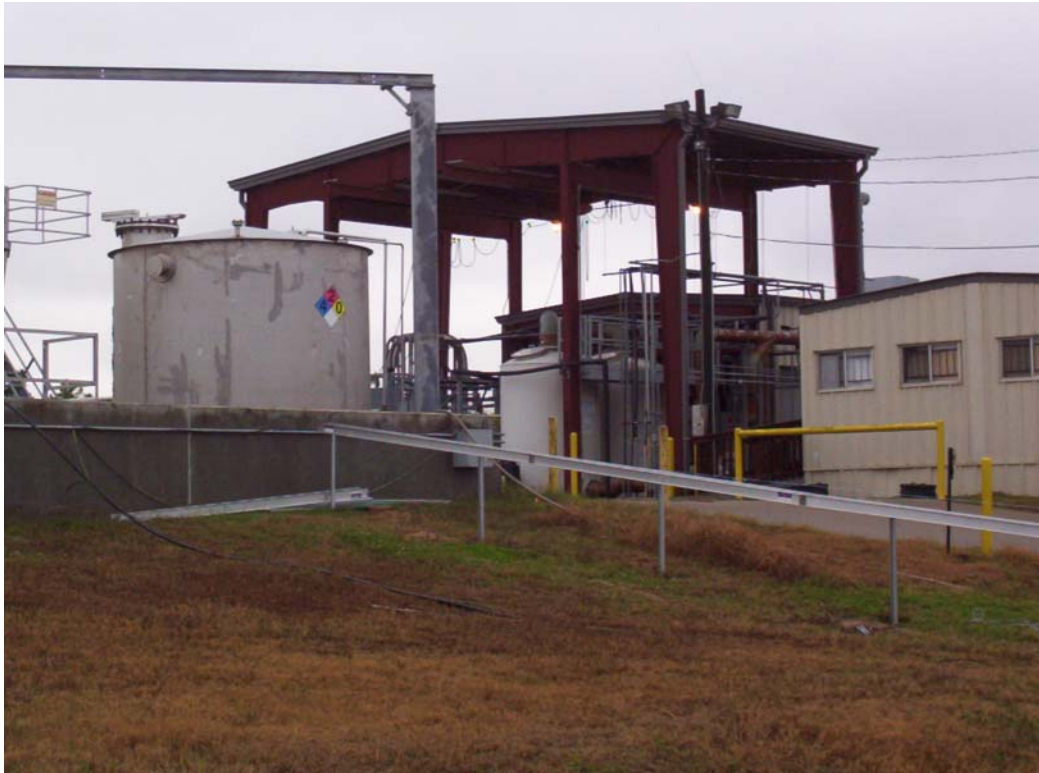
Photo 3. Facing west, DNAPL collection tank and southern ends of treatment plant and site office.
