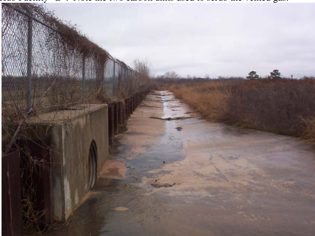
Photo 10. Inside fence line, facing west, looking up road/drainage pathway. Drainage outlet to Mud Gully on left. Note top of sheet pilings on left along fence line..
