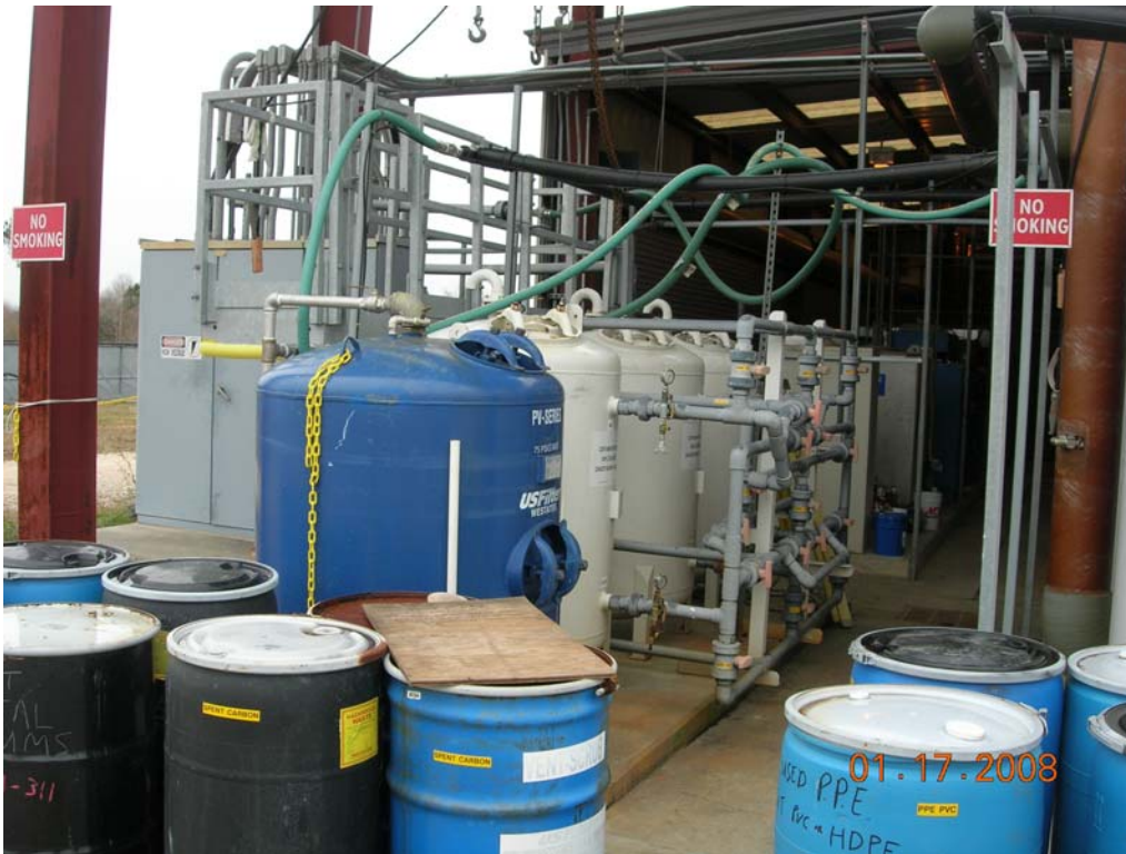
Photo 19. Looking into the treatment area. Blue tank is prefilter using carbon as filter material. Gray tank are carbon filters used to polish water after air stripper.
