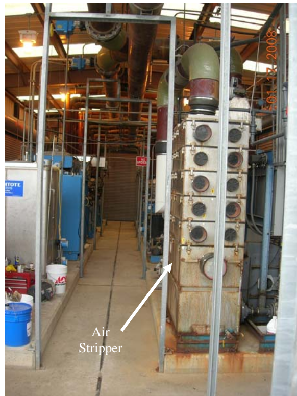
Photo 20. Air stripper with filters in Photo 19 to the photographer's back.
