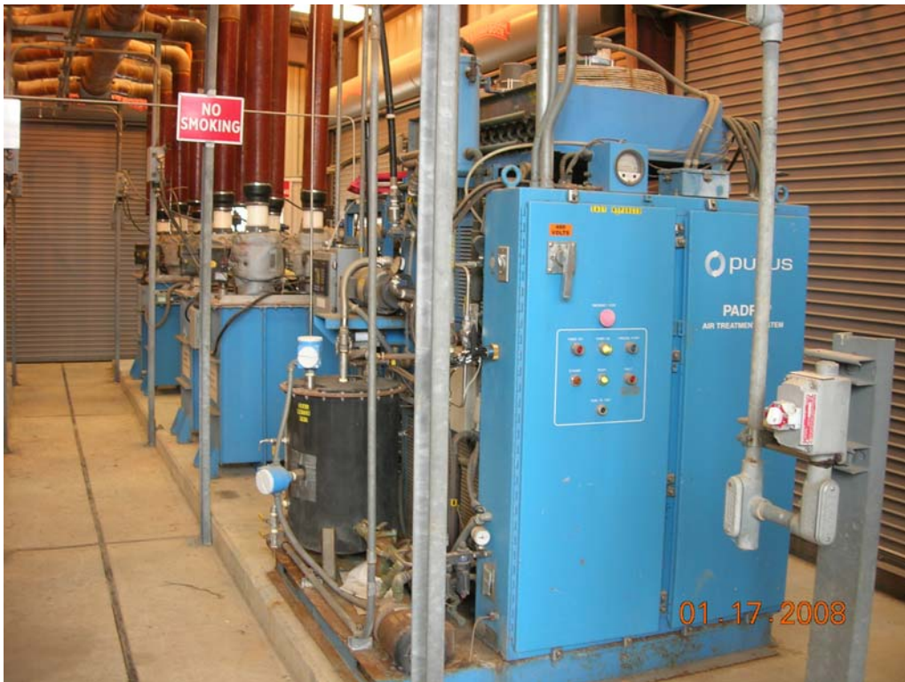
Photo 21. Post-stripper air treatment system. Units in background are solid resin bed adsorption units used to remove volatile contaminants removed by air stripper. Unit in foreground is vapor recovery system used for regeneration of resin beds.
