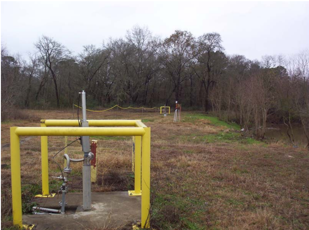
Photo 14. Facing southeast, Brio South plume wells, PO-610 and PO-613. Note Mud Gully on right side of photo.
