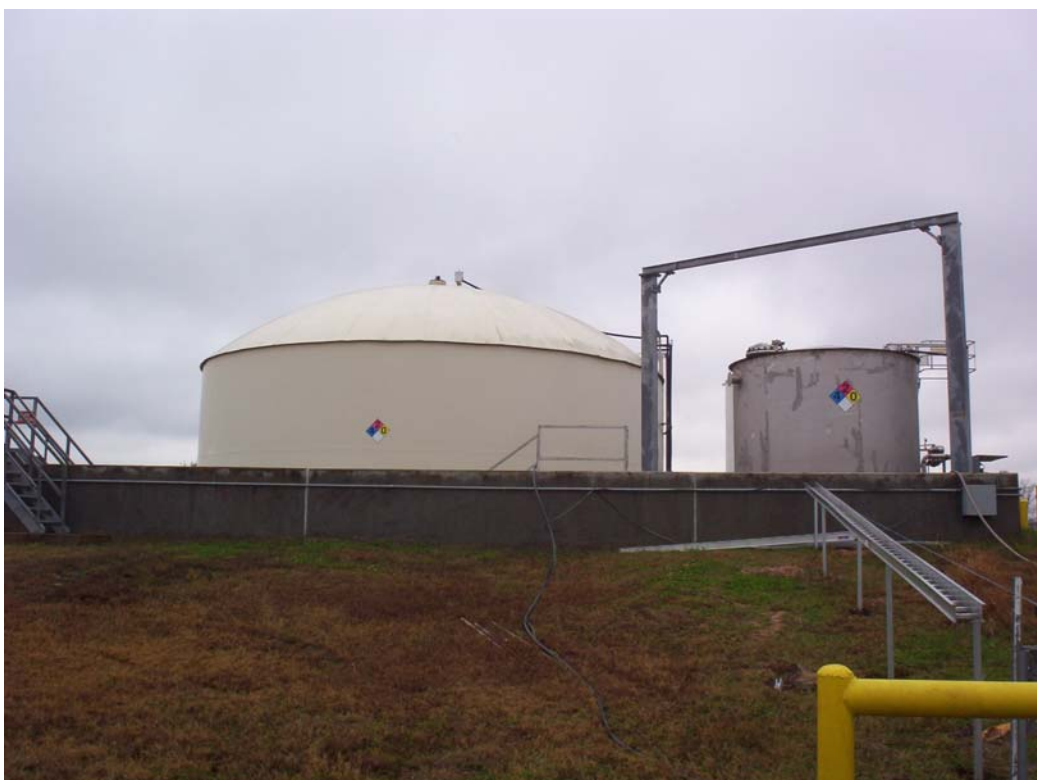
Photo 2. Facing southwest, groundwater collection tank (left) and DNAPL collection tank (right).
