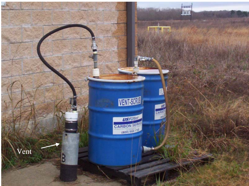
Photo 9. Gas Collection Vent on Compartment “B” located on southwest side of Hub Facility “B”. Note the two carbon units used to scrub the vented gas.
