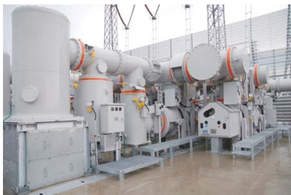
300 kV GIS 300 kV gas-insulated switchgear (GIS)
