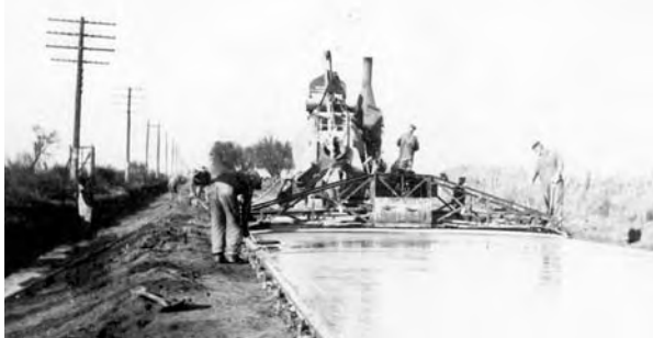
Paving the Lincoln Highway between Ames and Fremont in Dodge County, c.1920 (Photo courtesy of NDOR)
