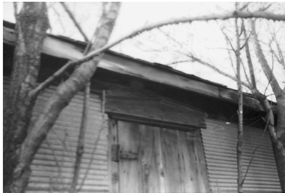
Photo 12– detail of door hood on former house (granary) looking northwest Photo by Dan Kidd, 1978, NSHS (7811/11:20)
