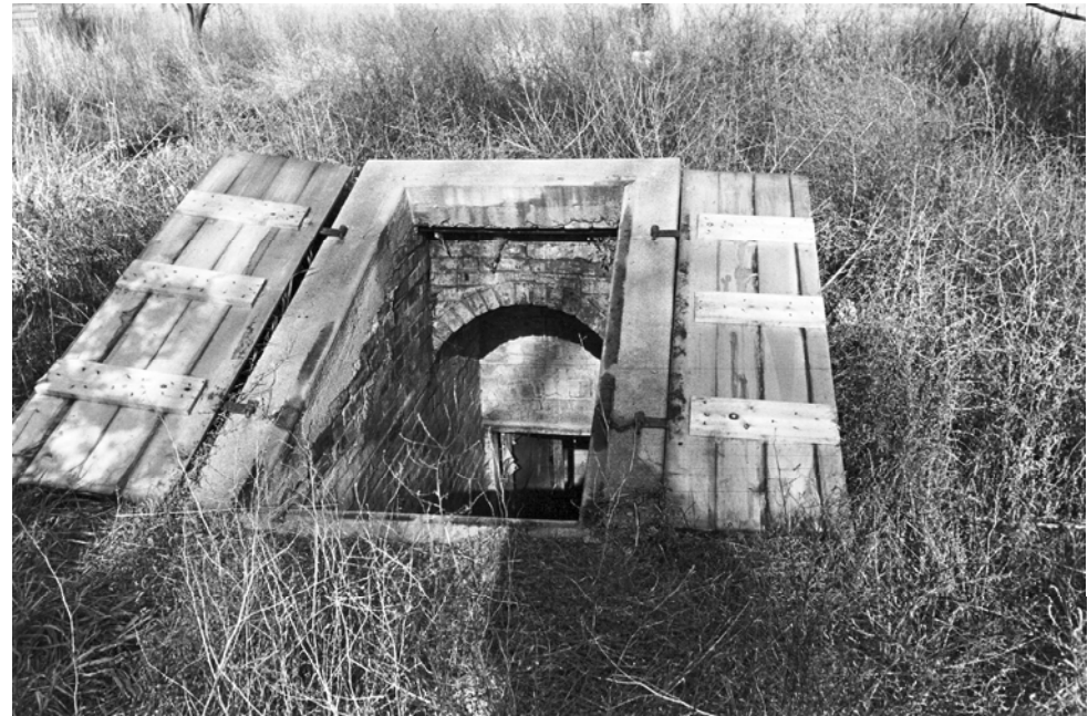
Photo 2– detail view of brick vaulted cellar looking east Photo by Dick Spencer, 1978, NSHS (7804/8:11A)
