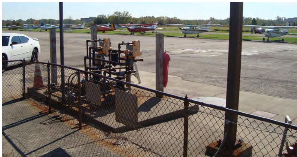
Fuel pumps and underground storage tanks near the Co-op Aviation building will be removed prior to the start of any park improvements.
