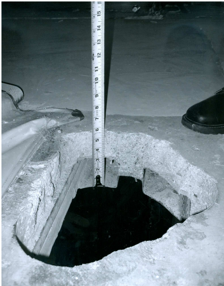
4th floor, typical wiring raceway
