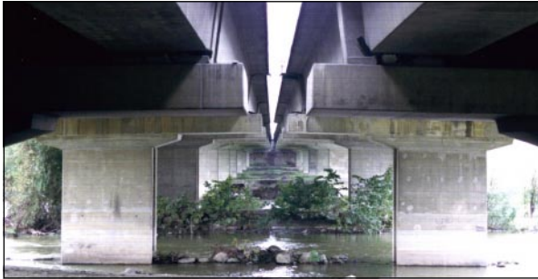
Figure 3. The east (left) and west (right) bound bridges over the Sakarya River. Note shifting of the spans and the unseating of the bearings in the west-bound bridge. The bearings on the east-bound bridge have partially "walked out," but not unseated.
