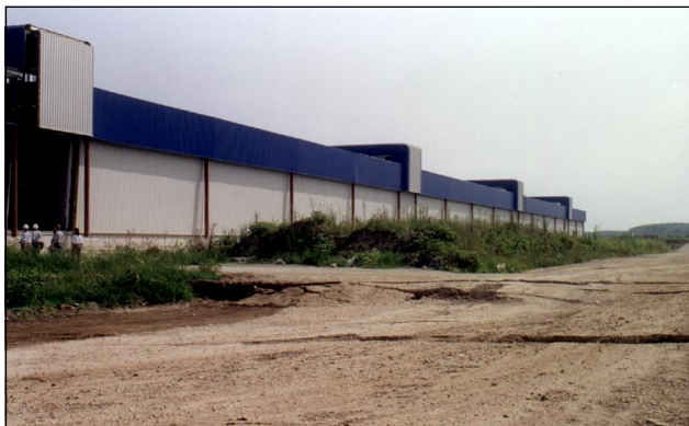
The fault rupture is visible next to this damaged manufacturing facility, under construction at the time of the earthquake.
