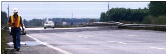
Figure 4. A typical view of the bump-onto-the-bridge on the E80 motorway. Up to 500 mm embankment settlements were common over a 20 km stretch of road. Notice the guard rail in the photograph as further evidence of the embankment settlement.
