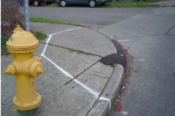
Walkway ready for curb ramp. Create stockpile of objects for embedment as curb ramps and new walks are established
