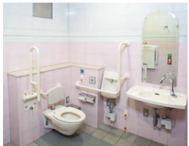
Multi-functional lavatories with ostomate facilities
