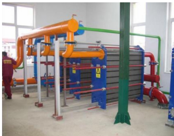
Geothermal distribution point, Romania
