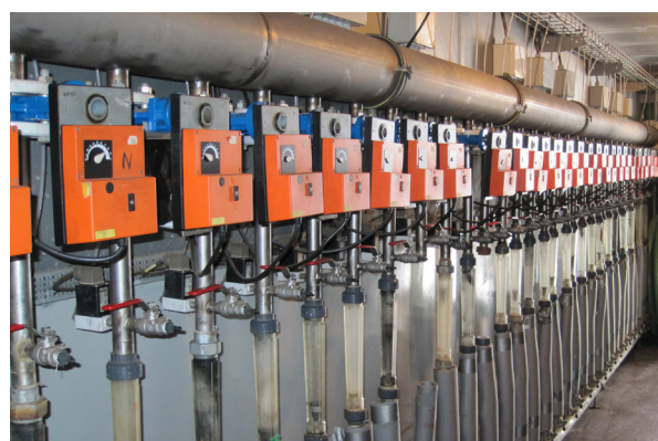
New methane gas works, Poland
