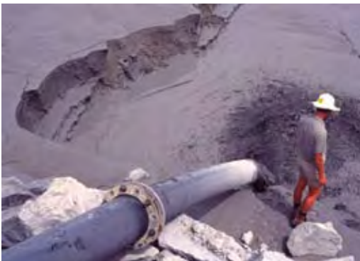
Conventional tailings slurry disposal
