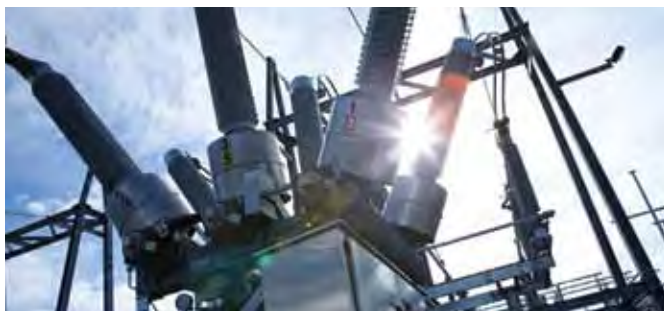
Above: Harewood West Substation, south of Nanaimo
