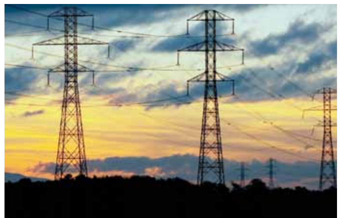
Above: Transmission lines 2L010 and 2L057 (double circuit) and 2L006 and 2L063 in Delta, B.C.
