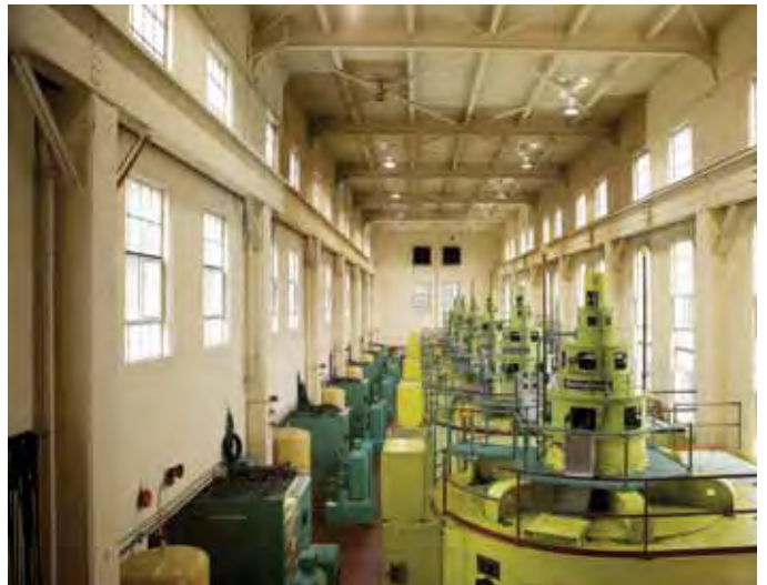
Above: John Hart Generating Station, Campbell River—2011
