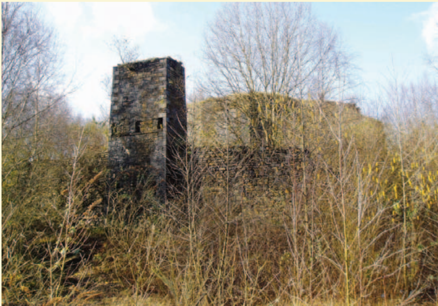
The Pier to the former waste tip tramroad is built into a boundary wall
