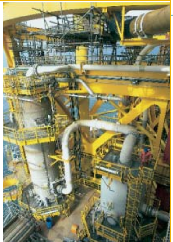
The treatment facilities. The gas is brought into contact with the solvent in a column called an absorber, thus increasing the gas/solvent exchange and the absorption of the acid gases.
