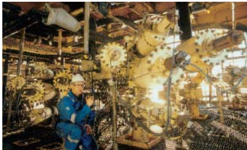
The wellhead area on the Elgin wellhead platform.
