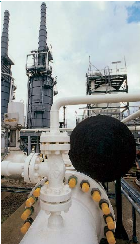
Newly built gas metering and heating facilities within the Bacton terminal (Norfolk).
