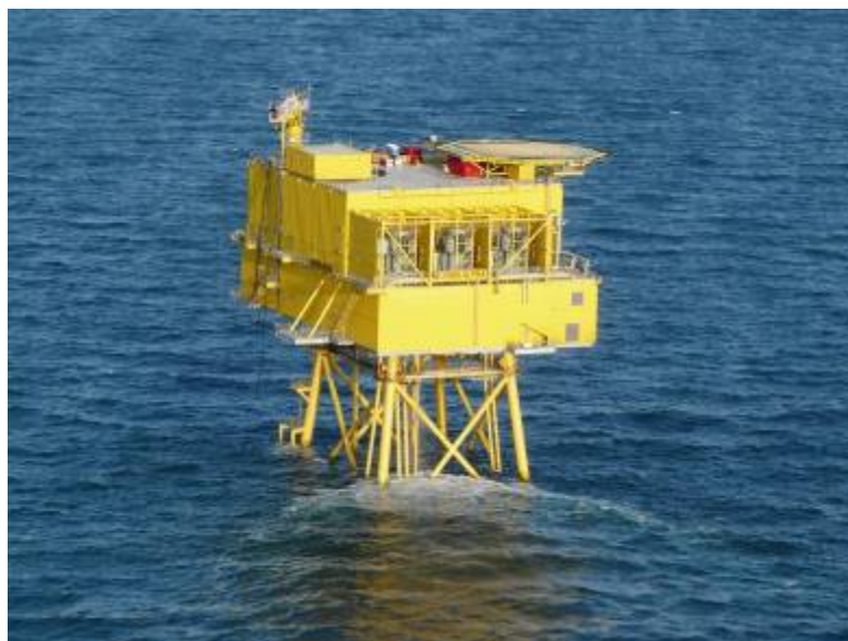
Fig 6. Offshore converter station BorWin alpha evacuates wind-generated power.
