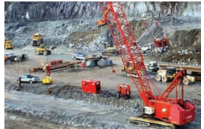
Local 302 operators are pictured here working on an ongoing dock project in Dutch Harbor, Alaska for West Construction.
