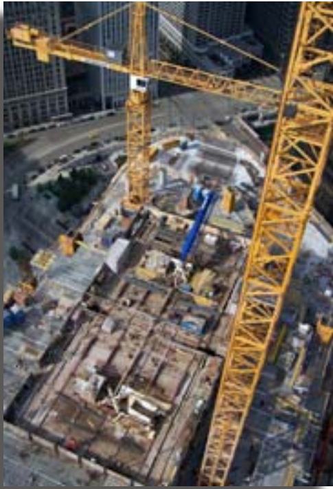
High above the Windy City, James McHugh Construction's Local 150 tower crane operators had a fantastic aerial view of the Trump Tower project.
