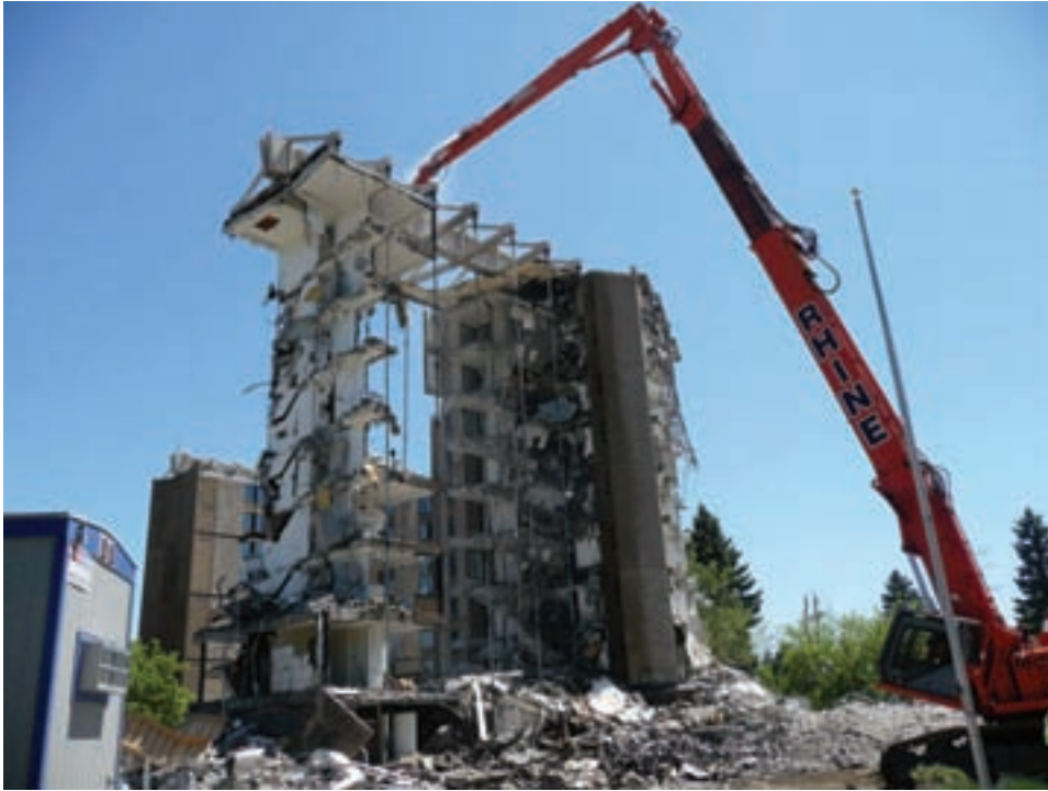
Operator Gil Olson, a 29-year member of Local 302, is seen here using a RW Rhine crane with a long-reach excavator to perform the demolition of the Courson and Muzzall Halls at Central Washington University in Ellensburg, WA for contractor Wm. Dickson.
