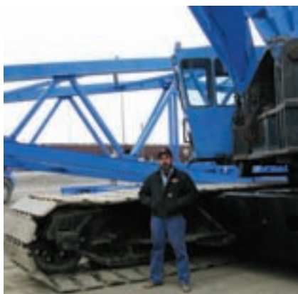
Lampson 4600 operator, Doyle "Bump" Jordan, said that this is the first 4600 ever built. They are using this crane to tear down the 2600.
