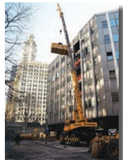
A Local 150 operator for Brandenburg Industrial Services hoists a box to remove debris from the Sun-Times building, which was demolished to make room for the Trump Tower.
