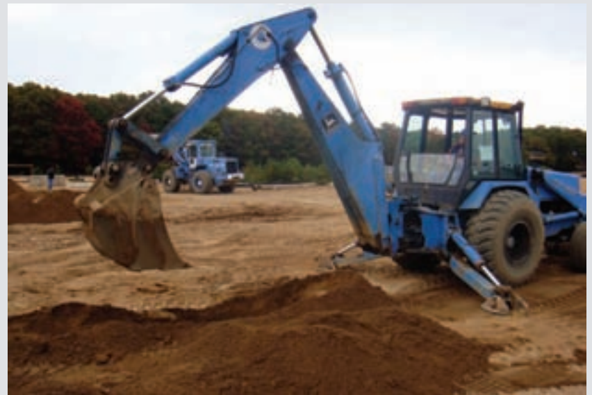
Local 138's Jose Vilaca, a second-year apprentice, digs a trench with a John Deere backhoe during Dirt Wars 2008.
