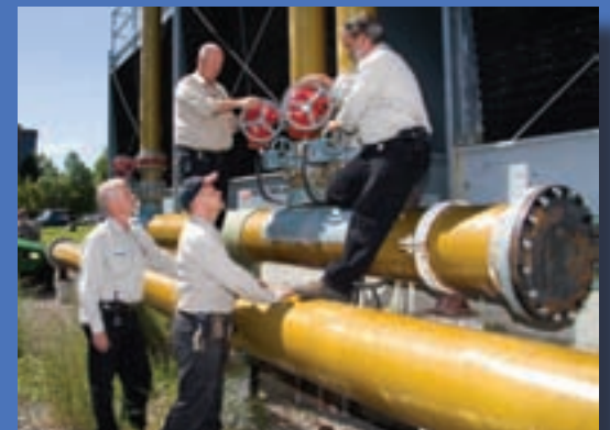
Local 865 stationary engineers at Lakehead University are pictured here taking Marley Cooling Towers out of service for seasonal maintenance.
