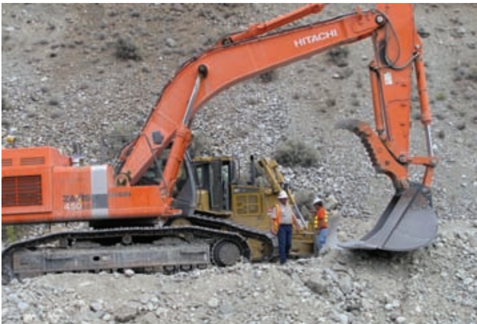
29-year Local 302 member Walt Madson II, left, served as job steward for contractor Goodfellow Bros. on the Chelan County PUD fish habitat project near the Chelan River in eastern Washington.
