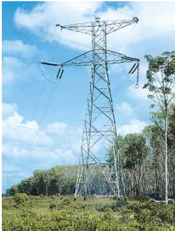
Fig. 5.6.1-1: DC transmission line (bipolar tower 300-kV link)
