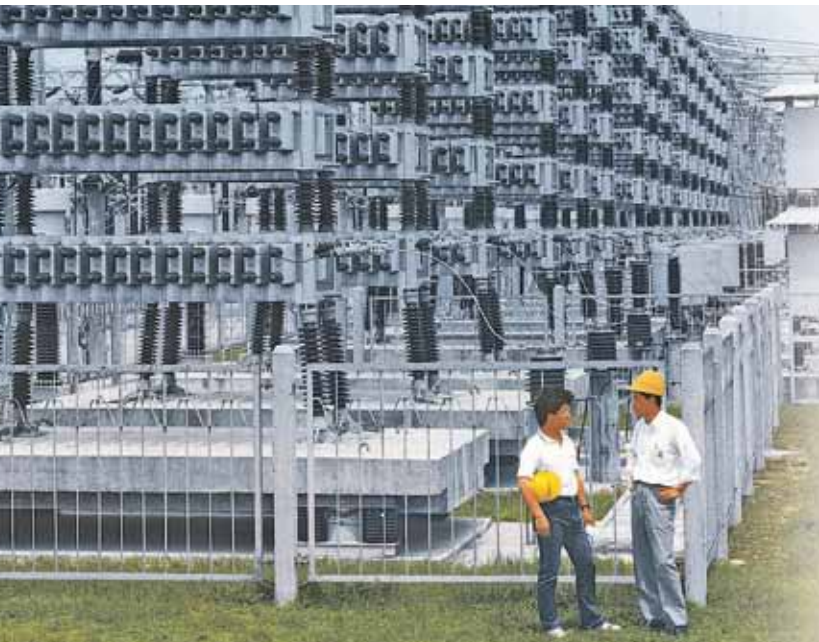
Fig. 5.4.1-2: AC filters and capacitor banks of Gezhouba/Shanghai
