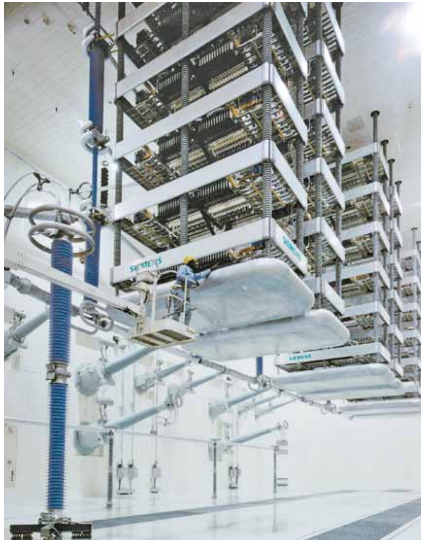
Fig. 5.1-8: Converter valves Sylmar HVDC station, Los Angeles, USA
