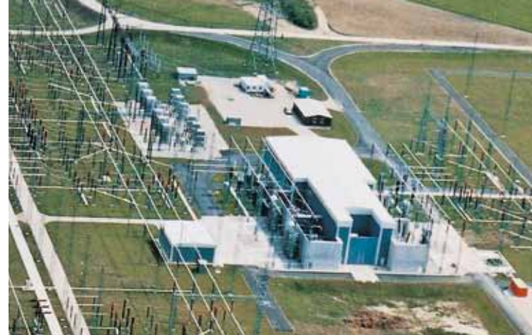
Fig. 2-3: Back-to-back converter Station Vienna Southeast
