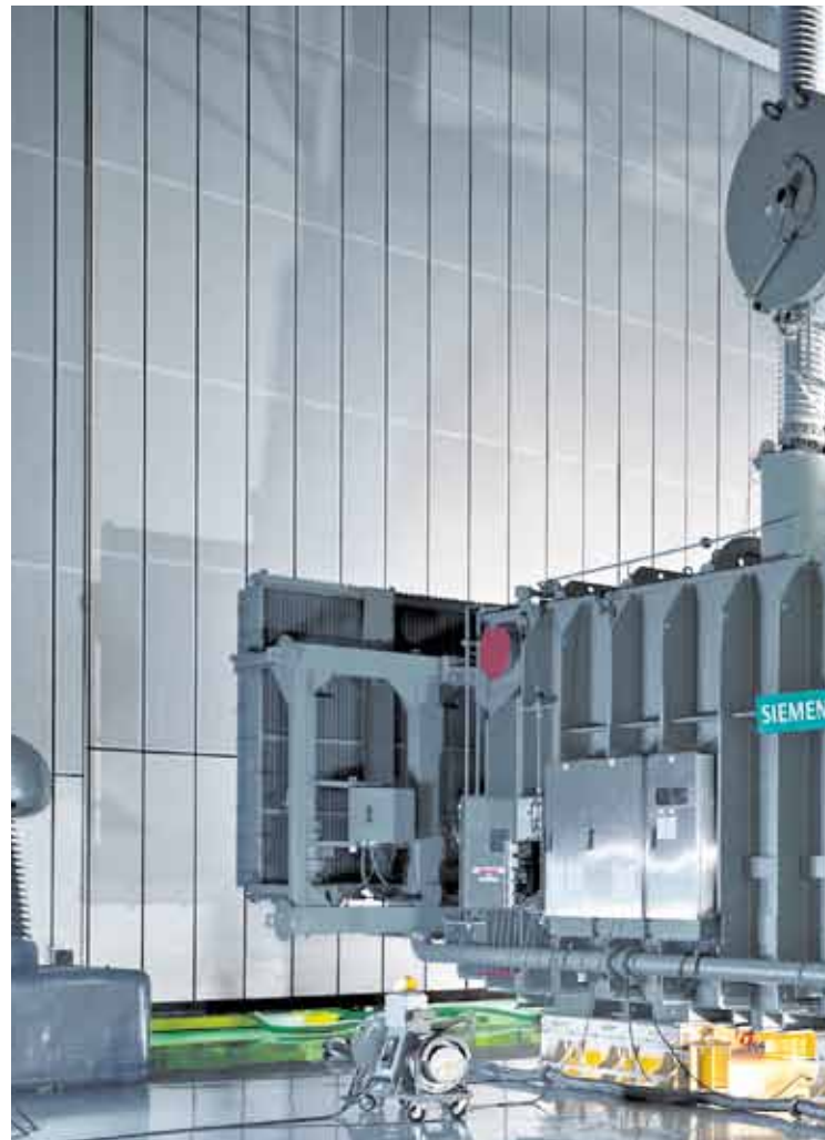
Converter transformer for the Three Gorges HVDC project 284 MVA, 1-ph/2-w unit
