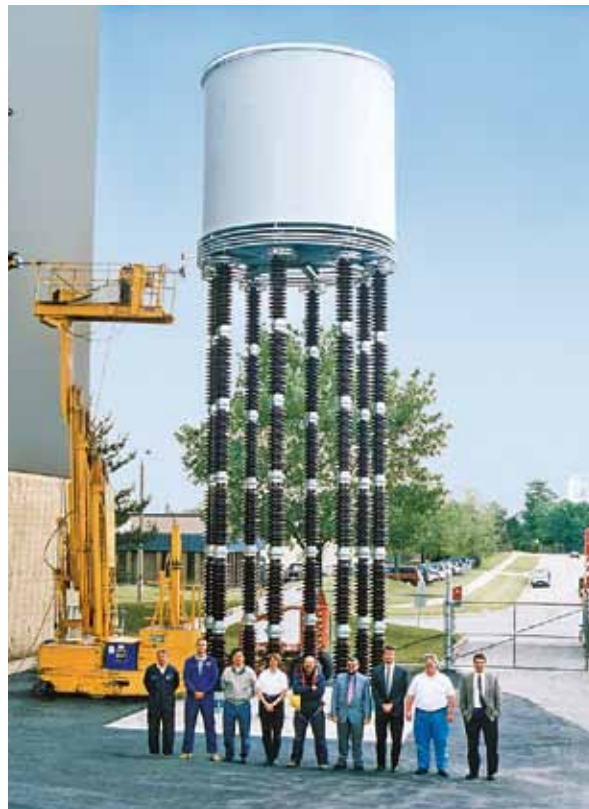
Fig. 5.3-2: Air-insulated smoothing reactor – Tian Guang project
