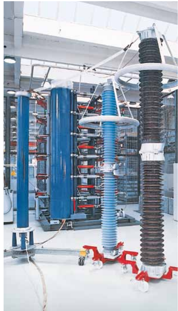
Fig. 5.5-2: Measurement of residual voltage on porcelain-housed (foreground) and polymer-housed (background) arresters
