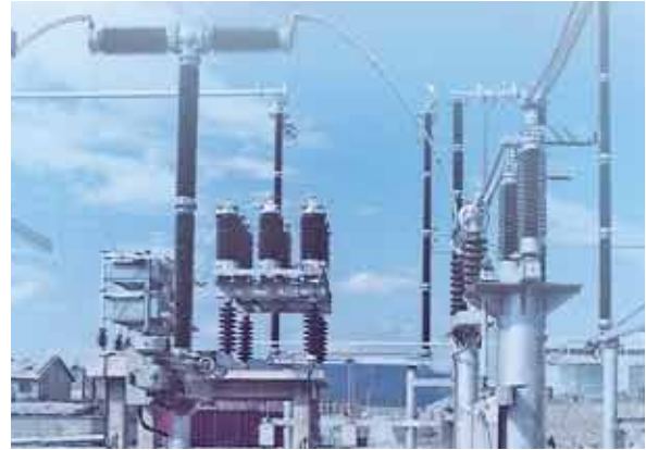
MRTB at Tian Guang/China DC switchyard
