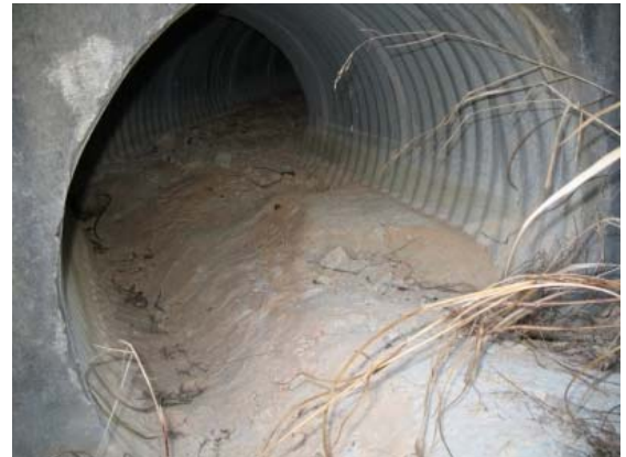
<Photo 1> Deposited sediment in water channel
